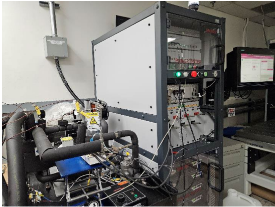
Figure 5. Photos of the module heat exchanger assembly piped into the dielectric fluid loop and electrically connected to the PowerTester
